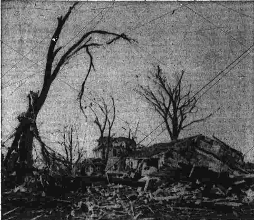
These homes in Waseca, Minn., show the effects of tornadoes that ripped through the area yesterday. Several persons were killed, many more injured and damage was estimated in the millions. (AP Photofax)
